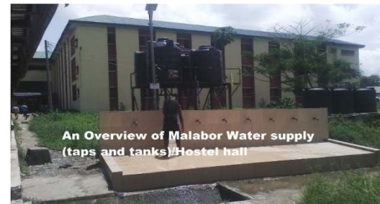
Photo 3. An overview of the Malabor hostel water supply
