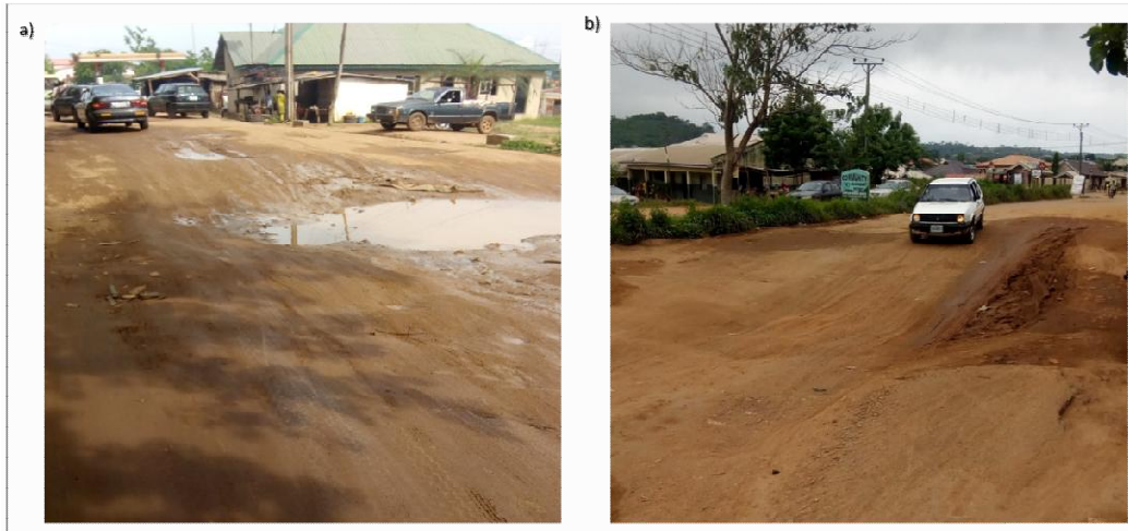
Fig. 1. a) Failed portion of the Apete-Akufo Road Southwestern Nigeria. (b) Failed portion of the Apete-Akufo road, with hills covered in vegetations showing in the background
