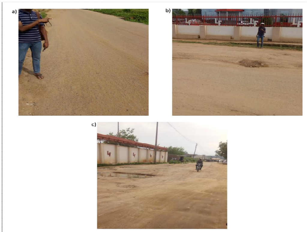
Fig. 5. a) Stable (b) Unstable and (c) Highly Unstable sections of the Apete-Akufo road
